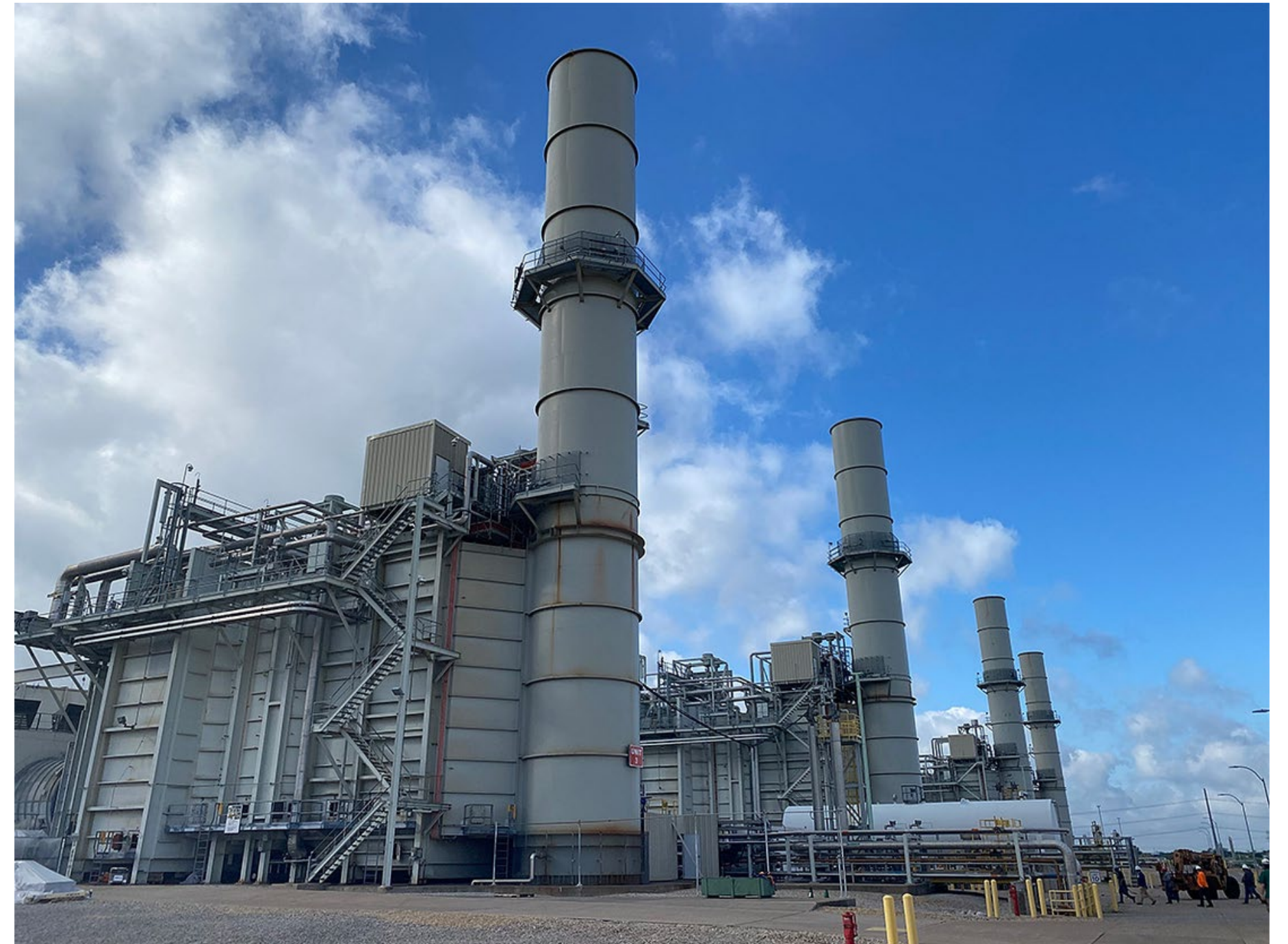
Midlothian Power Plant
